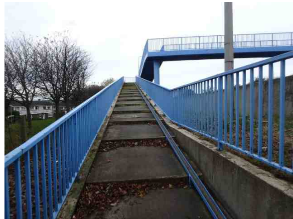
F.7 – A photo taken on the western side of North Dene Footbridge
