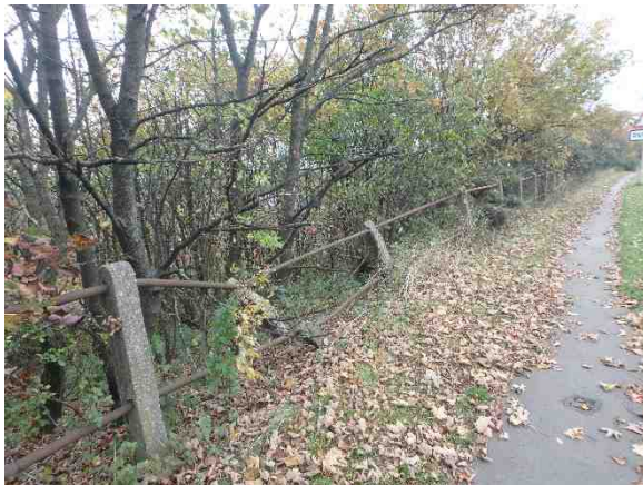
F.3 – A photo focusing in on the fencing on the western side
